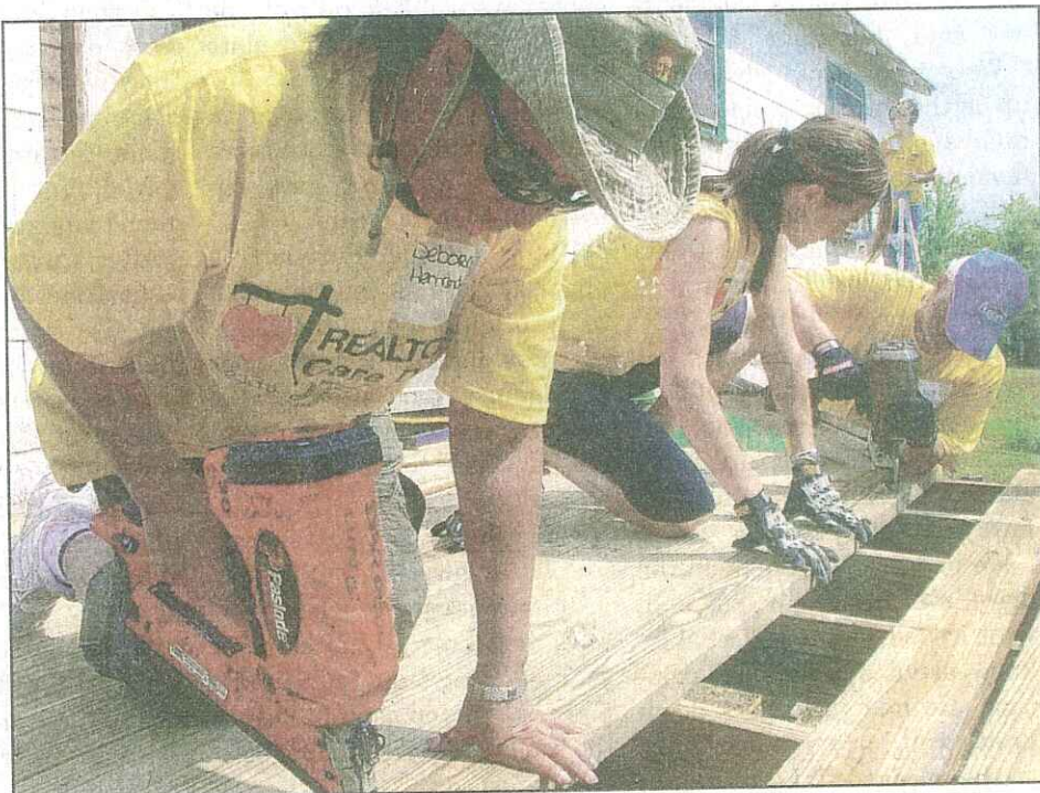
Deborah Hernandez (left) of Reed Realty in Charlotte, helped Sheena Sutton and J.D. White of Coldwell Banker United in Mooresville, build a small deck where a crumbling rear porch used to be.
